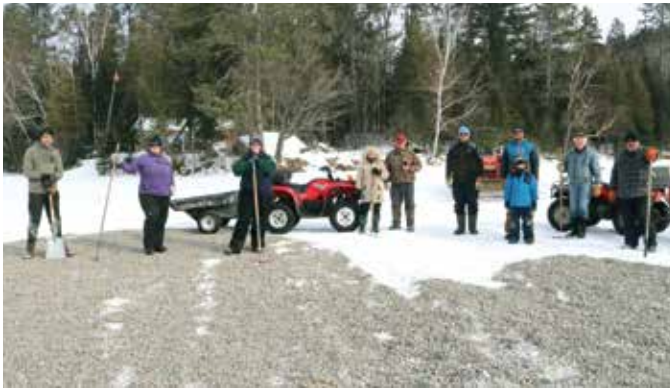
Completed walleye spawning bed project on Diamond Lake near Killaloe. A You-Tube clip is available through Watersheds for more details.
